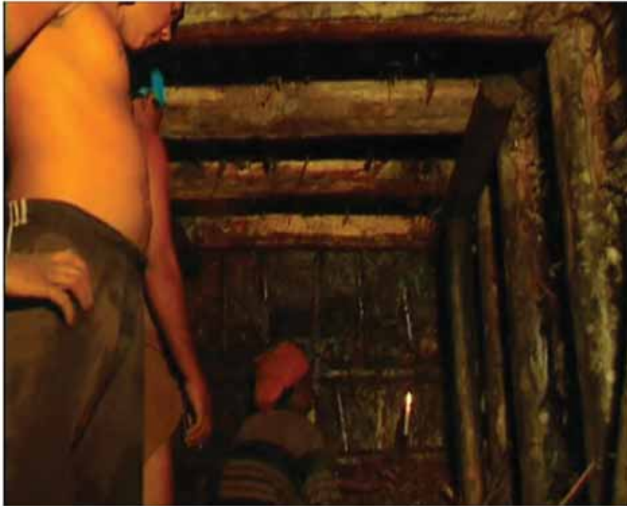
Propping up the walls with beams and rafters to prevent them from caving in.
